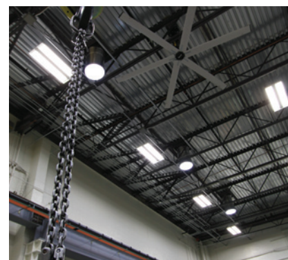
What seemed "to good to be true" is now a fixture at Stardust Roller Rink. Pictured above is the MacroAir 24' AirVolution in action.
